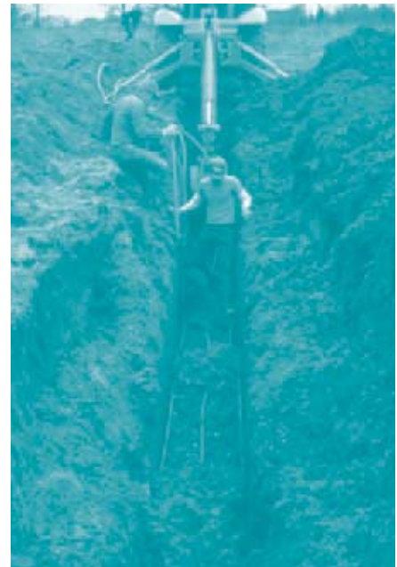
A backhoe is used to dig a horizontal trench for laying a ground loop.
